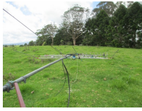
VHF & UHF antennas going together
